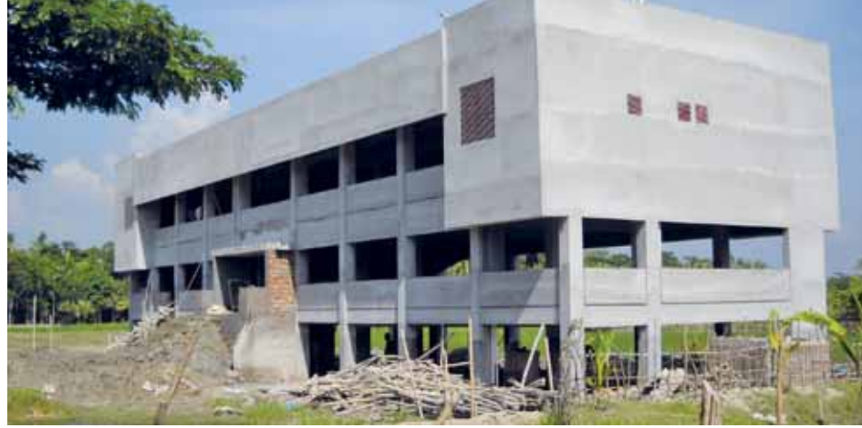
A shelter under construction with SDC support. Location: Hogolpati, Bangladesh Photo credit : F. Poffet
